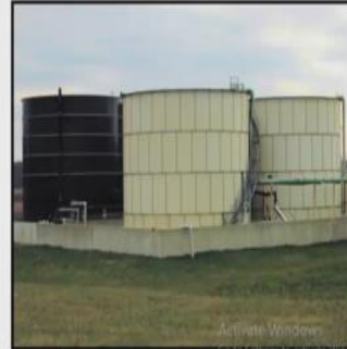
Glass lined steel leachate storage tank
