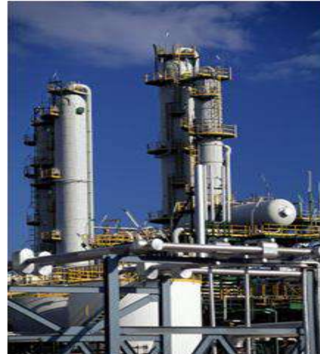
Flue Gas Desulfurization System
